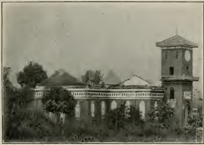
RUINS OF THE CHURCH AT LIEN-CHOU. Burned by the Mob, Oct. 28, 1905. The tower still stands.
